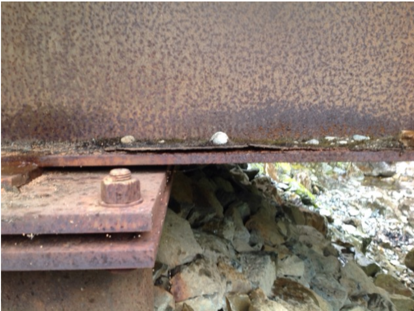
minor delamination of bottom flange
