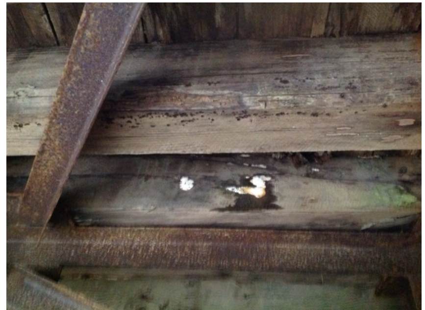
ties showing signs of decay - up to 40%
